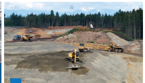
7 Shaping and compacting of stockpile 2. The new access road to the landfill will run alongside stockpile 2.
